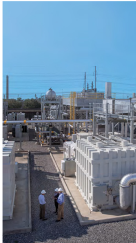
FuelCell Energy reports its 14.9MW fuel cell platform in Bridgeport, Connecticut, has provided clean and reliable power since 2013.
