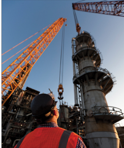
In 2011, our Baton Rouge chemical plant installed new facilities to further expand feed flexibility.
