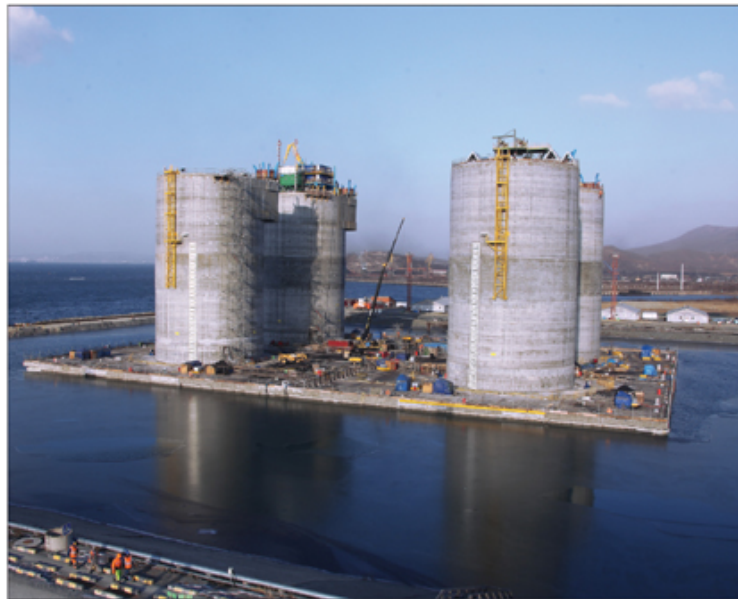
We achieved mechanical completion of the Arkutun-Dagi offshore platform concrete gravity-based substructure (GBS) in December in far east Russia.
