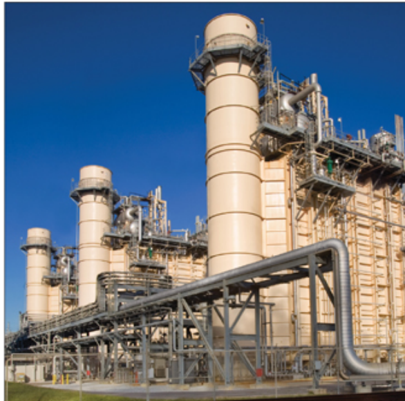
Cogeneration provides a significant source of efficient energy for our refining and chemical sites.
