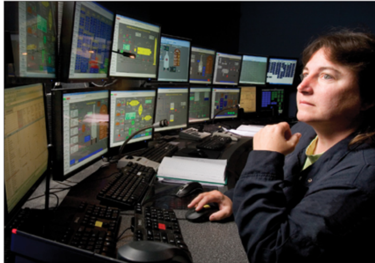
Specialized training and well-equipped control rooms are essential components of operational excellence.
