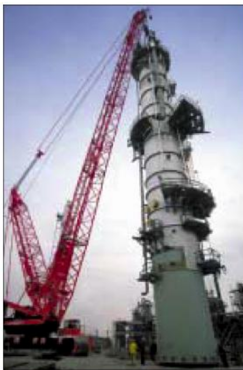
Installation of the naphtha splitter fractionation tower at the Joliet, Illinois, refinery for production of low-sulfur motor fuel.
