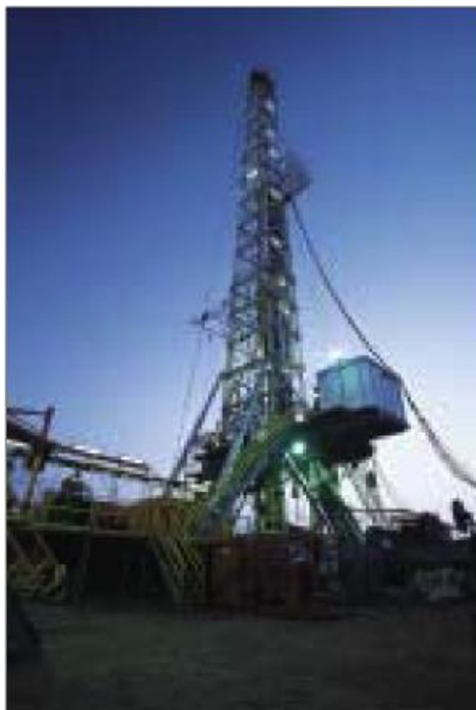
Drilling one of the 265 wells needed for the 1-billion-barrel (gross) Doba development in Chad. Early production is expected in 2003.
