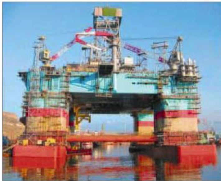
Construction of semi-submersible drilling rig at Baku, Azerbaijan. The rig will be the largest and most powerful unit in the Caspian Sea. The first well to be drilled with this rig will be on the ExxonMobil-operated Zafar Mashal block in 2003.
