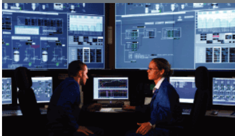
Advanced control systems, such as the computer controls for our plastics plant in Meerhout, Belgium, coupled with implementation of best practices and operations discipline result in efficient operation of our facilities.
