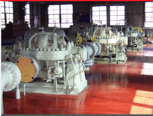
New pumps being installed at the Conway, Arkansas, pump station as part of the project to expand capacity of the Pegasus Pipeline.
