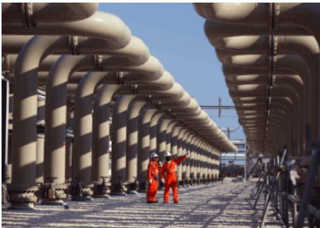
In 2009, ExxonMobil and our joint venture partner, Qatar Petroleum, started up three 7.8-million-tonnes-per-year LNG trains, the largest in service anywhere in the world.
