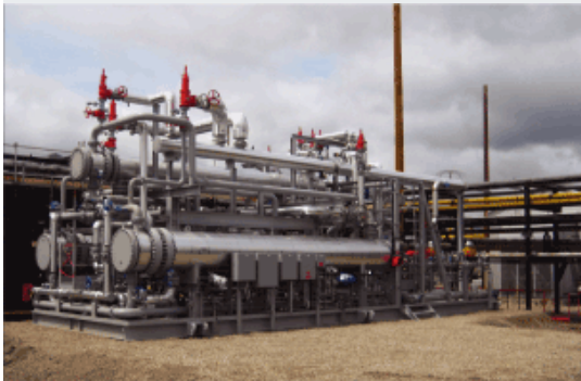
This testing equipment was installed at the West Pembina field in Canada to conduct a field trial of ExxonMobil's proprietary ColdFlow technology, which combats the formation of hydrates.
