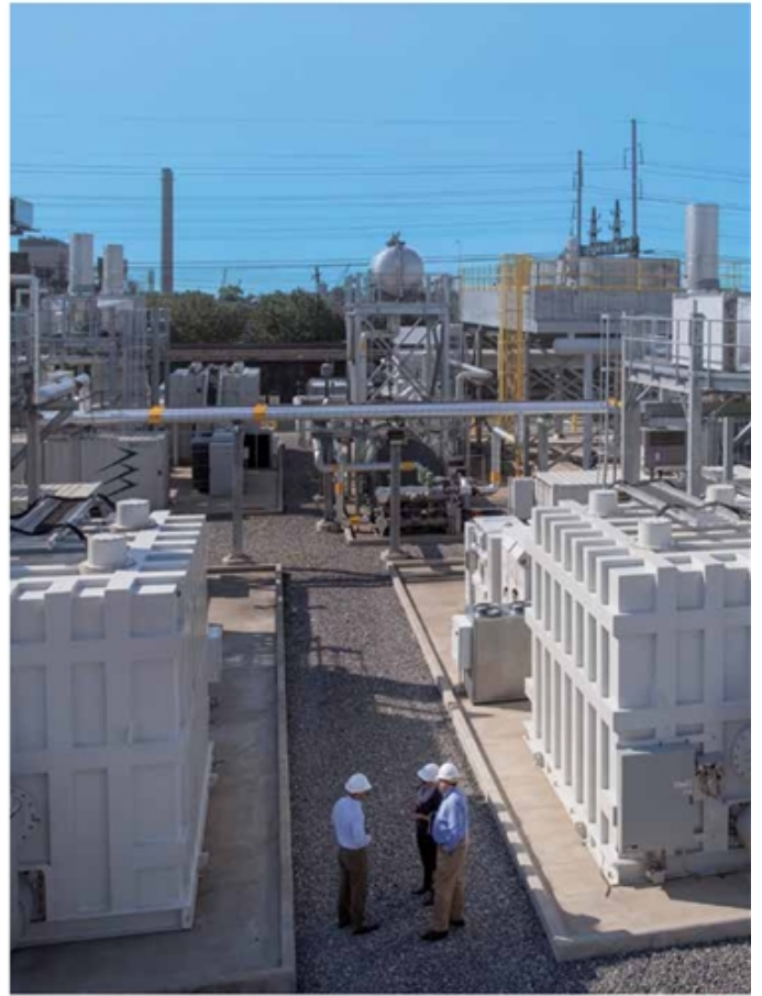
→ FuelCell Energy reports its 14.9MW fuel cell platform in Bridgeport, Connecticut, has provided clean and reliable power since 2013.
