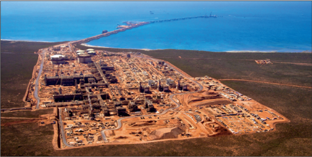
The LNG plant construction and commissioning continues on Barrow Island for the Gorgon Jansz project in Australia.
