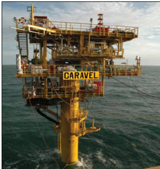
The joint-venturer-operated Caravel field in the U.K. North Sea is being developed with a monotower design.
