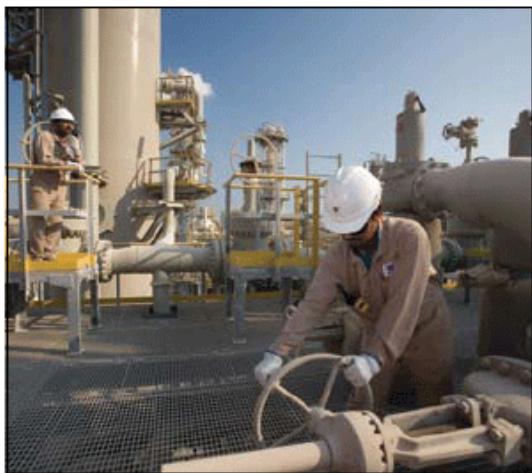
Production of LNG from Ras Laffan Liquefied Natural Gas Company II Train 5, shown at left, began just 29 months after major construction contracts were awarded.
