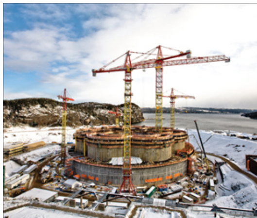
The Hebron project, which will utilize a gravity-based structure (shown under construction), will have gross production capacity of 150 thousand barrels per day and will be located in 300 feet of water offshore Newfoundland.
