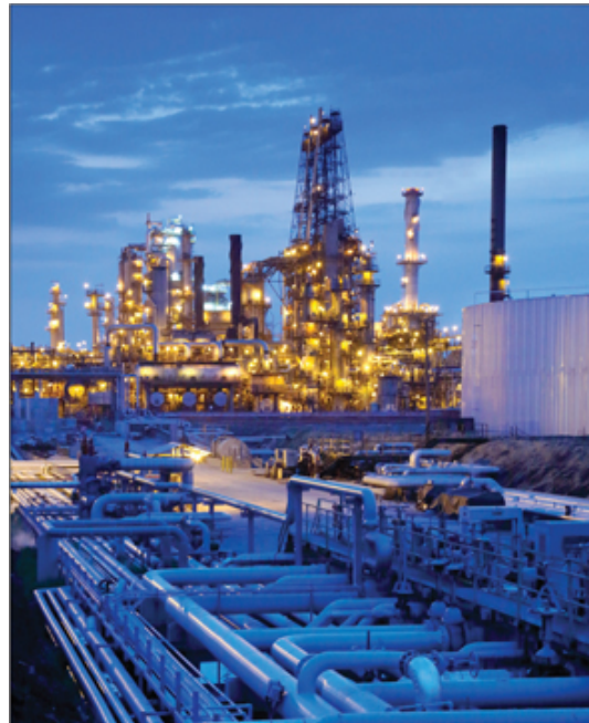
ExxonMobil is an industry leader in feedstock flexibility and challenged crude processing. For example, our Joliet Refinery is able to process significant volumes of lower cost, heavy Canadian crude.
