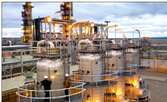
ExxonMobil is installing additional compression systems to increase sales of carbon dioxide and constructing a demonstration plant using the proprietary Controlled Freeze Zone technology at the Shute Creek plant in Wyoming.
