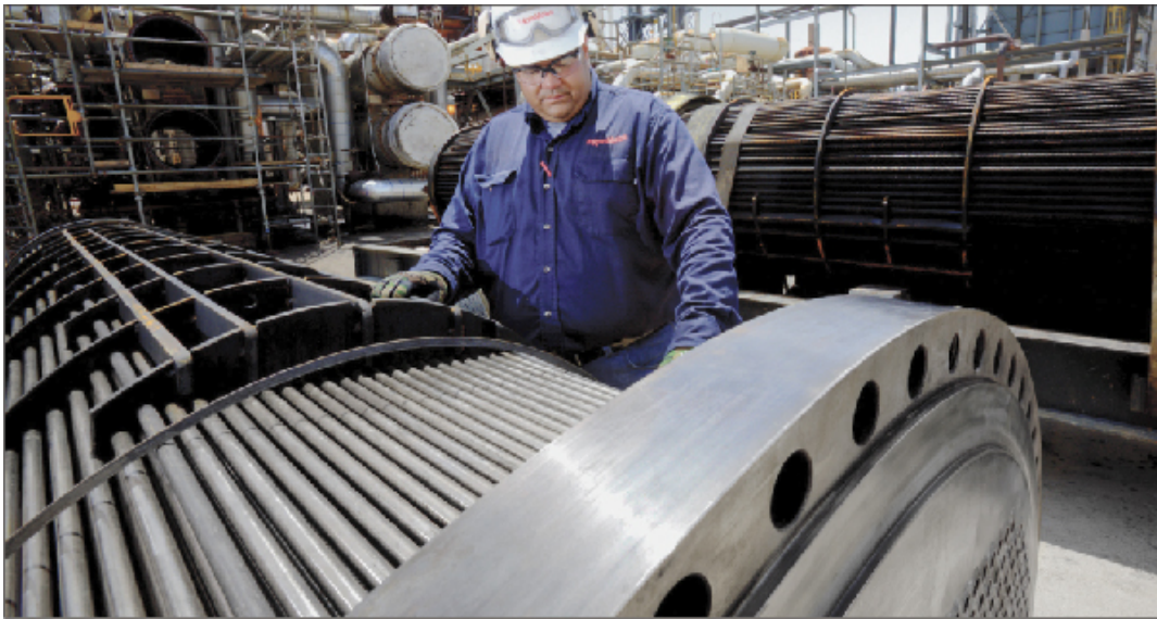
An engineer inspects a modified heat exchanger tube bundle prior to installation at a U.S. Gulf Coast refinery.
