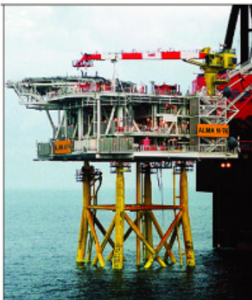
Installation of the Alma platform, part of the second phase of Sable Offshore Energy Project gas developments. This design will also be used for South Venture, scheduled to start up in 2005.
